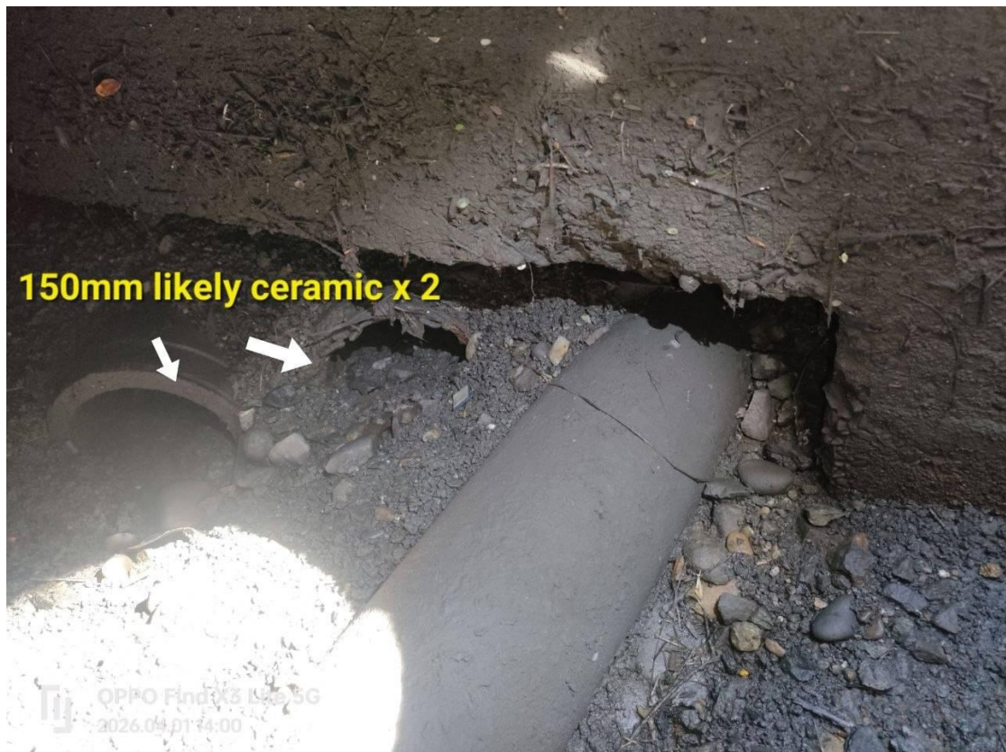
Figure 11: Stormwater chamber High Street Motueka
