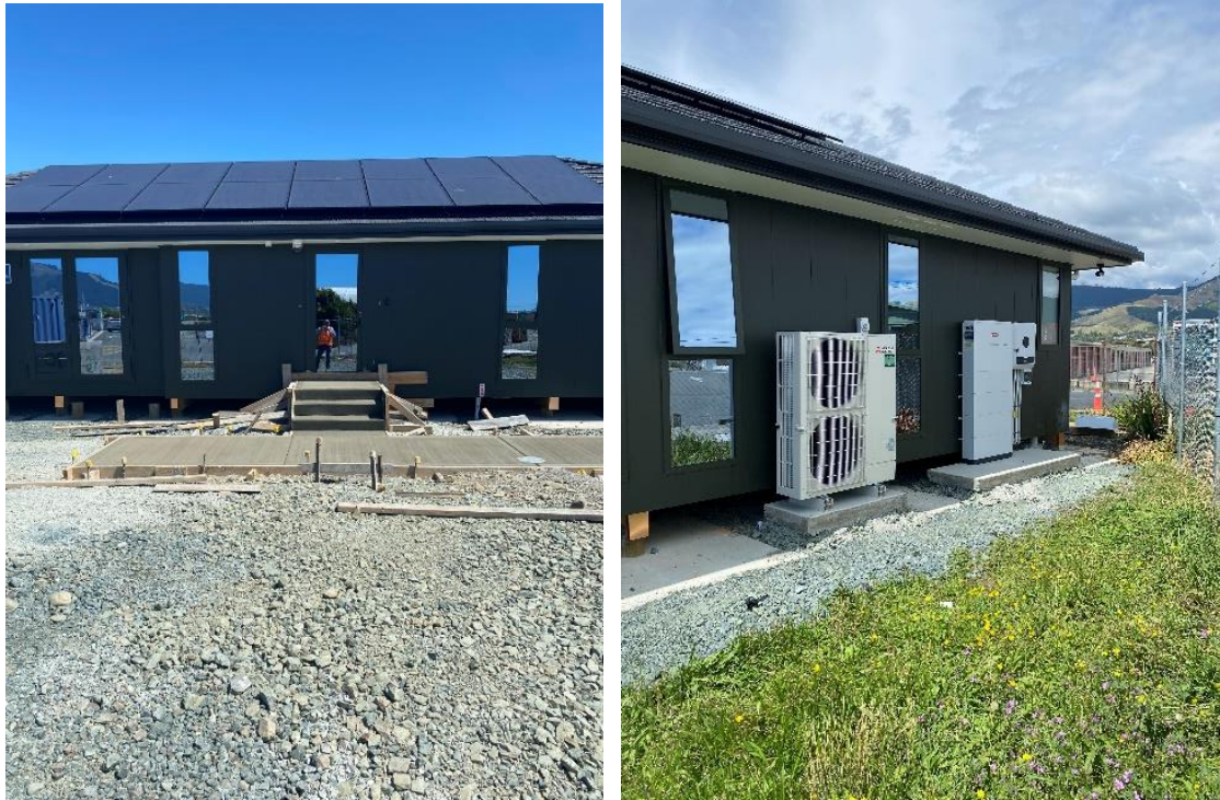
Figures 4 and 5: Richmond Resource Recovery Centre - new office path and steps and solar and battery system
