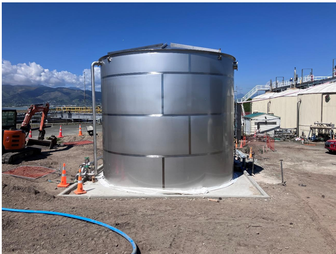
Figure 5: New Bell Island sludge storage tank
