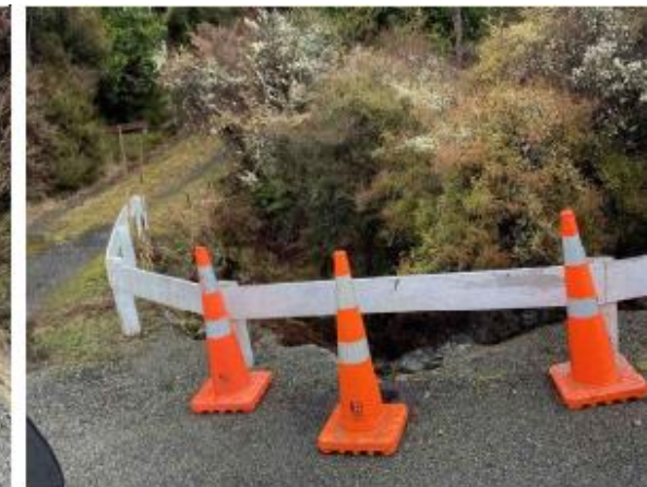
Borlase Avenue - sinkhole
