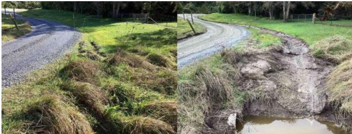
Rangihaeata Road – blocked culvert
