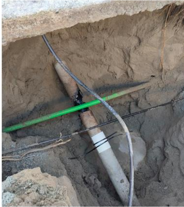
Figure 2: Fibre Optic Cable (green) strike on sewer pipe in Broadsea Avenue.
