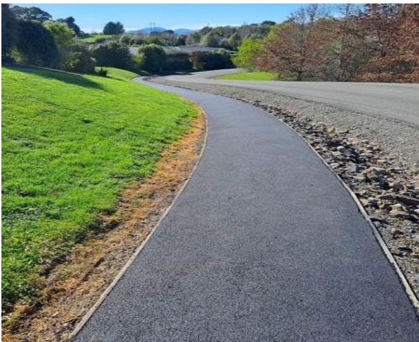
Picture 32- Ridgeview Road – Newly asphalted footpath. This path is approximately 900 metres long.
